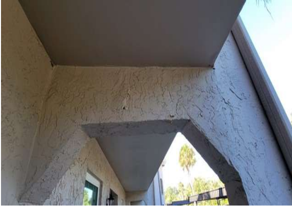
67 Damaged Stucco 1st Floor Near Unit 401 Overview
