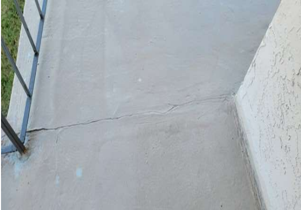
35 Cracked Walkway 2nd Floor Near Right Stairwell Overview
