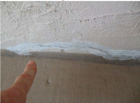
Level 3 Prior Repair For Separation at Walkway to Building Connection (Leaning)
