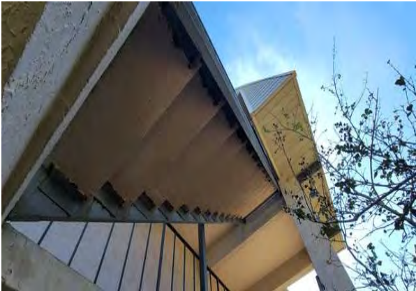
83 Rusted Tread Supports Stairs to 2nd Floor Front Right of Building Overview
