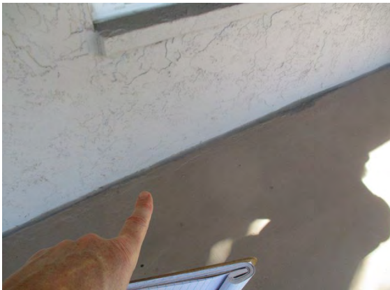
29 Level 2 Prior Repair For Separation at Walkway to Building Connection (Leaning)
