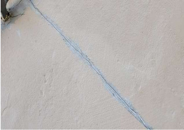
27 Cracked Walkway Near Elevator Lobby 3rd Floor
