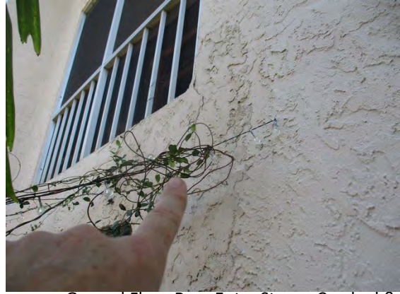
52 Ground Floor Rear Entry Stucco Cracked & Bulging
