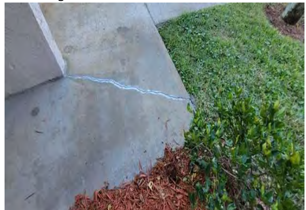
72 Cracked Sidewalk Front Right Corner of Building Overview
