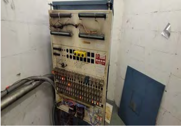
91 Elevator Control Board
