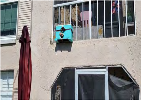
75 Cracked Stucco Rear Wall Between Units 401 & 501 Overview
