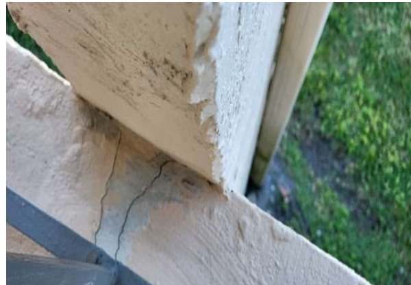
32 Cracked Walkway Near Unit 603
