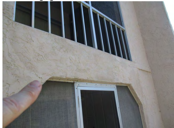
54 Ground Floor Rear Entry Stucco Cracked & Bulging
