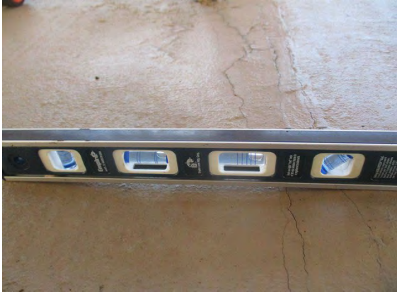
43 Level 2 Walkway Shifted/Displaced/Leaning Left Side of Building
