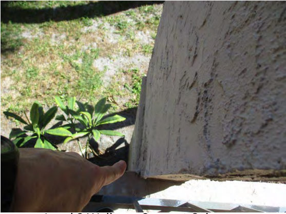
33 Level 2 Walkway Support Column Shifted/Displaced Left of #202
