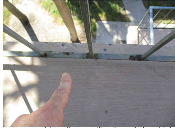
Level 3 Walkway Railing Corroded Multiple Areas
