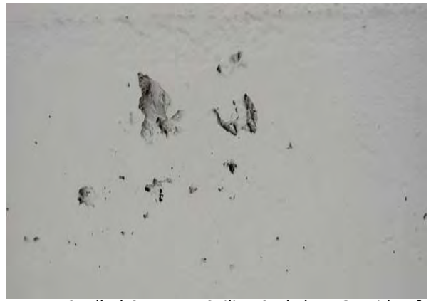
50 Spalled Concrete Ceiling 2nd Floor Outside of Electrical Room
