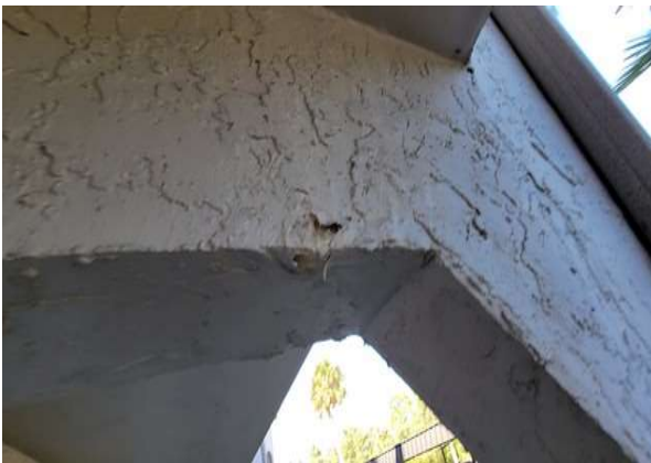
69 Damaged Stucco 1st Floor Near Unit 401
