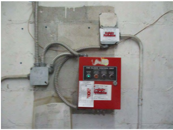
9 Fire Control Panel
