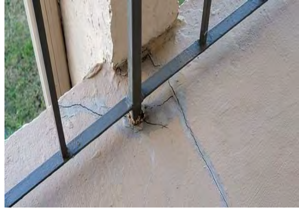
28 Cracked Walkway Near Elevator Lobby 3rd Floor
