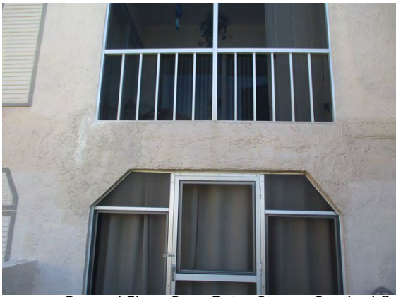
57 Ground Floor Rear Entry Stucco Cracked & Bulging
