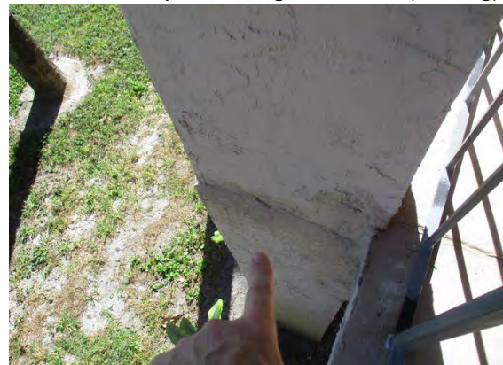
32 Level 2 Walkway Support Column Shifted/Displaced Left of #202
