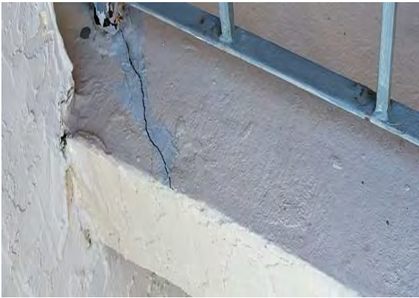
29 Cracked Walkway Near Elevator Lobby 3rd Floor
