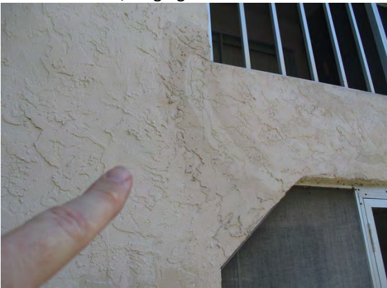
53 Ground Floor Rear Entry Stucco Cracked & Bulging
