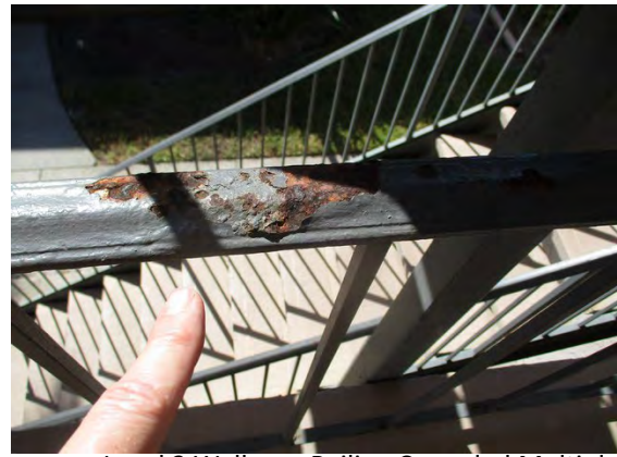
26 Level 2 Walkway Railing Corroded Multiple Areas
