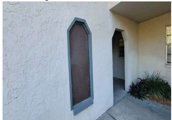
70 Broken Decroitive Window at 1st Floor Lobby Right Side Overview
