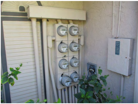
88 Building 8605 Meters & Main Panel
