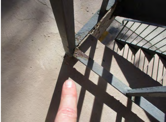
27 Level 2 Walkway Railing Corroded Multiple Areas
