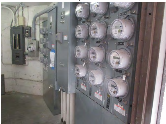
7 Meters & Main Panels
