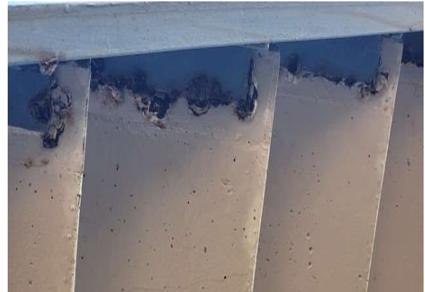
84 Rusted Tread Supports Stairs to 2nd Floor Front Right of Building
