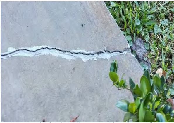
73 Cracked Sidewalk Front Right Corner of Building
