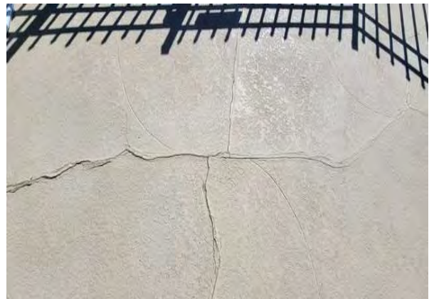
78 Cracked Pool Deck
