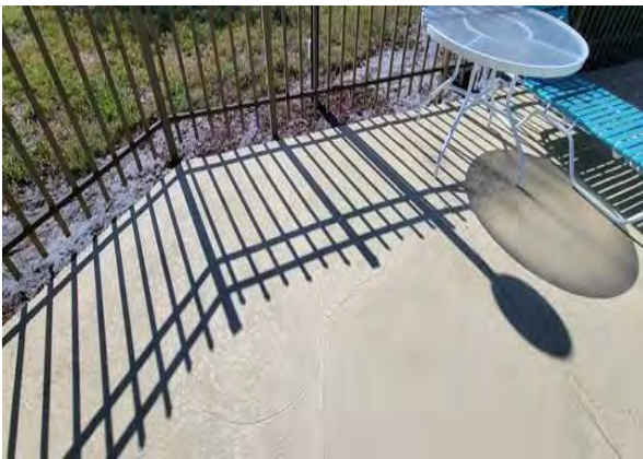
77 Cracked Pool Deck Overview
