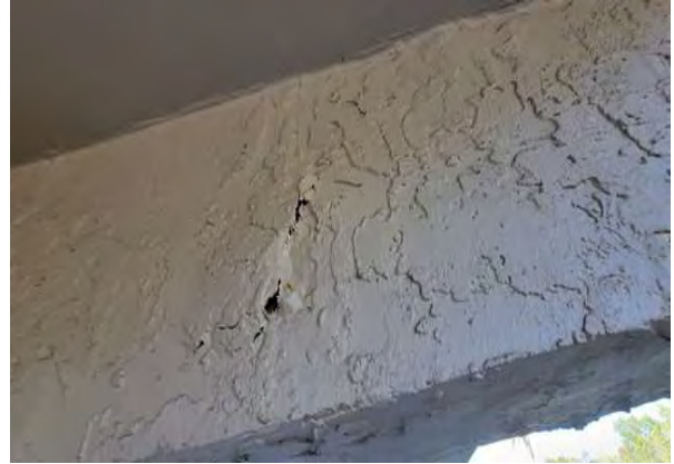
68 Damaged Stucco 1st Floor Near Unit 401
