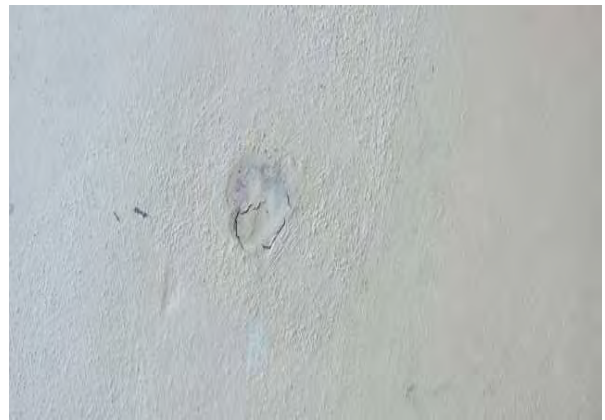
54 Damaged Concrete 2nd Floor Between Units 503 & 504
