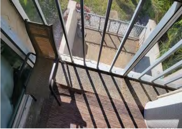
11 Unit 503 Balcony Cracking Overview
