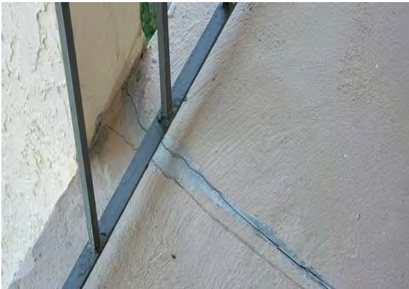
31 Cracked Walkway Near Unit 603
