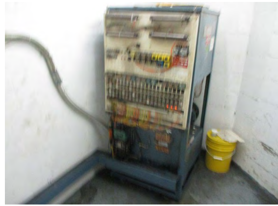
10 Elevator Control Board
