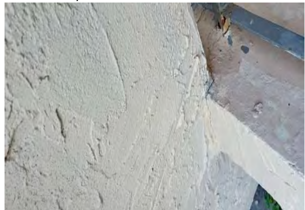
48 Cracked Walkway 2nd Floor Left of Elevator Lobby
