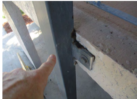
24 Right Stairwell Support Column Corroded
