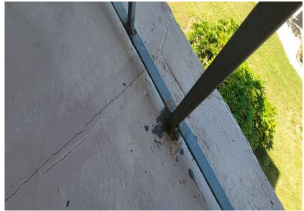
14 Cracked Walkway 3rd Floor Near Unit 608
