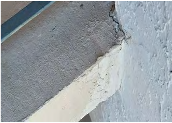
25 Cracked Walkway Near Unit 604
