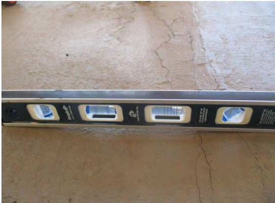
43 Level 2 Walkway Shifted/Displaced/Leaning Left Side of Building
