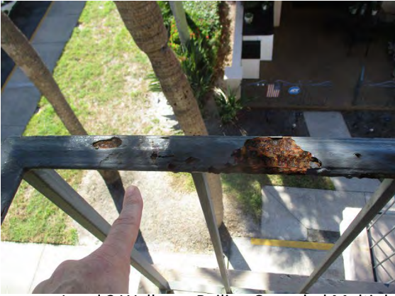
Level 3 Walkway Railing Corroded Multiple Areas
