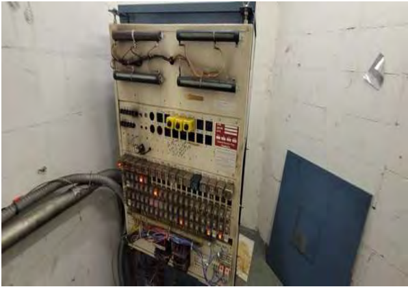
91 Elevator Control Board
