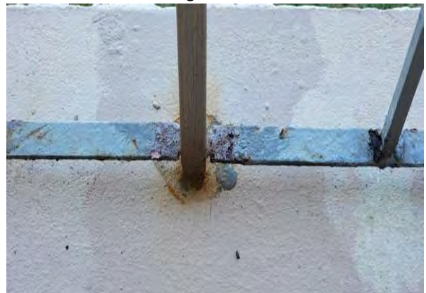
40 Rusted Handrail 2nd Floor Near Elevator Lobby Right Side
