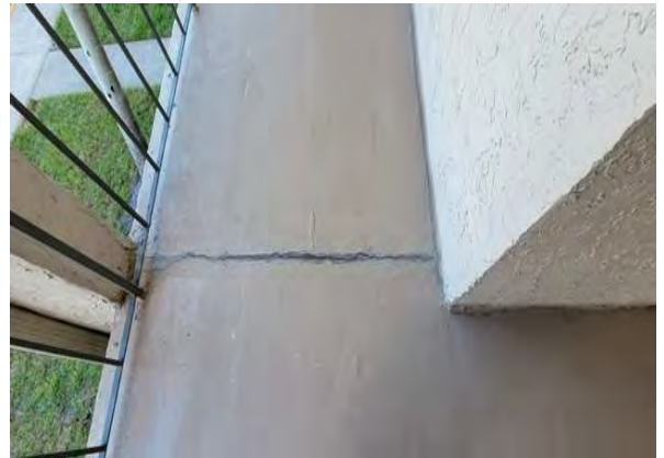
46 Cracked Walkway 2nd Floor Left of Elevator Lobby Overview
