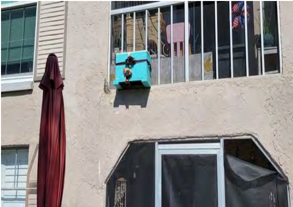
75 Cracked Stucco Rear Wall Between Units 401 & 501 Overview
