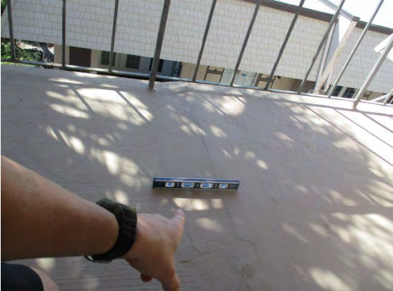
Level 3 Walkway Settled/Leaning At Left Side of Building
