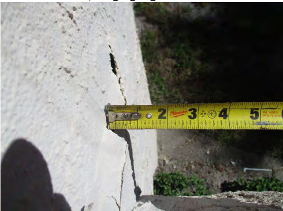
37 Level 2 Walkway Support Column Stucco Cracked/Bulging ~3/4" Right of #206
