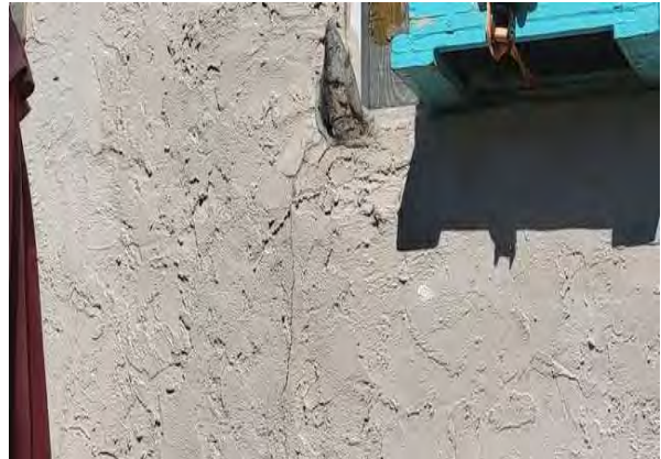
76 Cracked Stucco Rear Wall Between Units 401 & 501
