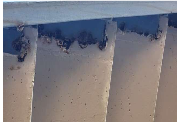
84 Rusted Tread Supports Stairs to 2nd Floor Front Right of Building
