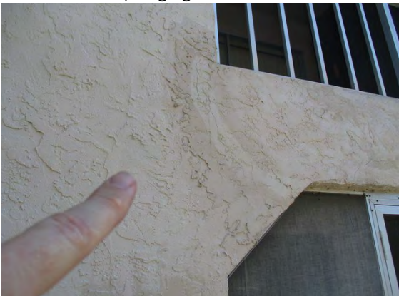
53 Ground Floor Rear Entry Stucco Cracked & Bulging
