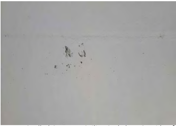
49 Spalled Concrete Ceiling 2nd Floor Outside of Electrical Room Overview
