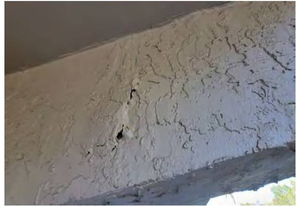
68 Damaged Stucco 1st Floor Near Unit 401
