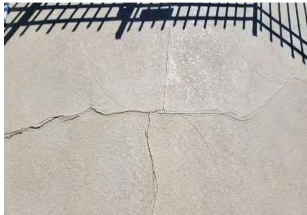
78 Cracked Pool Deck
