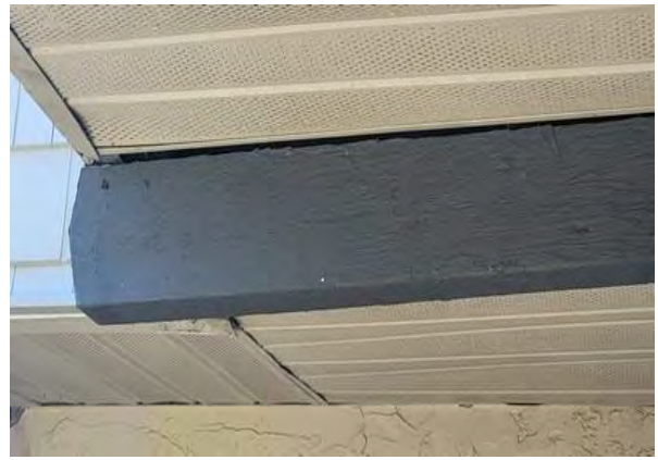
34 Sagging Support Member Near Left Stairwell
