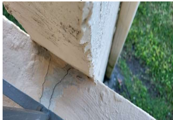
32 Cracked Walkway Near Unit 603
