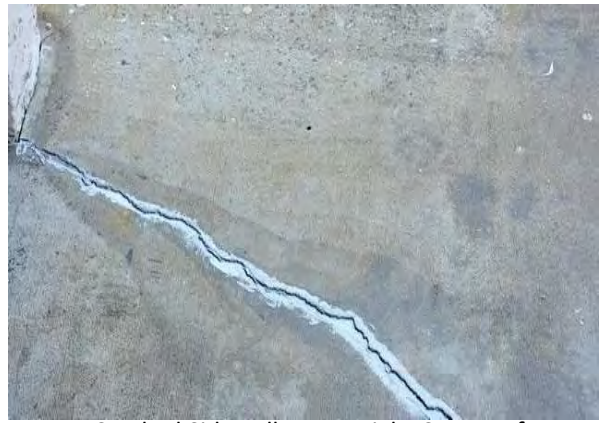
74 Cracked Sidewalk Front Right Corner of Building
