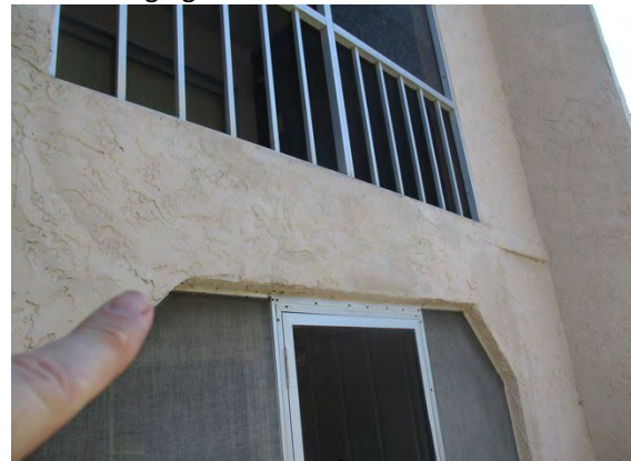
54 Ground Floor Rear Entry Stucco Cracked & Bulging
