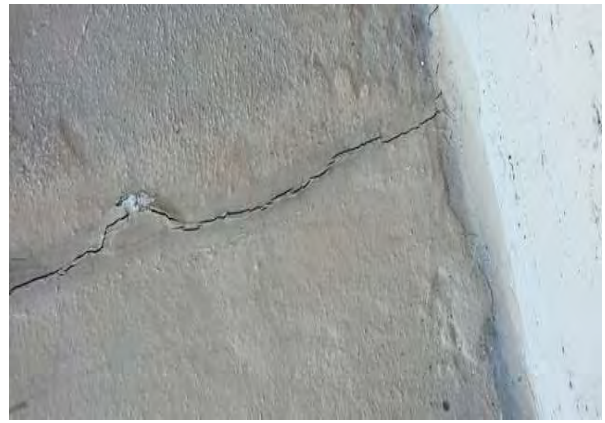
42 Cracked Walkway 2nd Floor Near Unit 504
