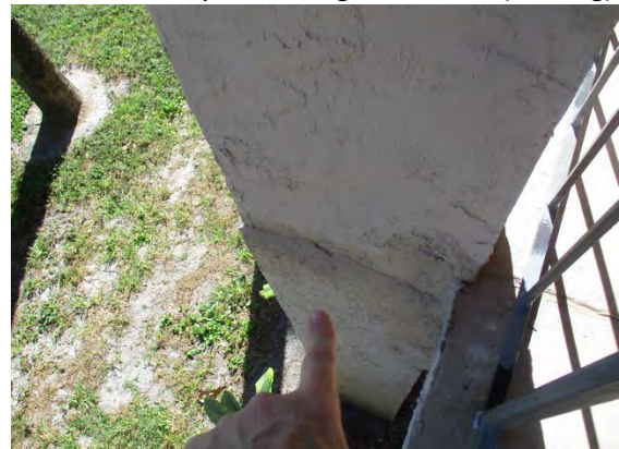
32 Level 2 Walkway Support Column Shifted/Displaced Left of #202
