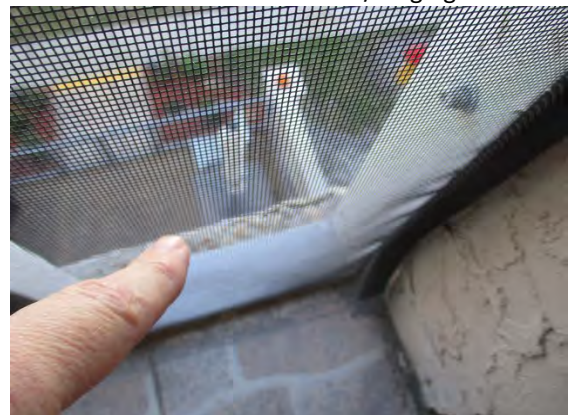
8 Unit 308 Stucco Cracked/Bulging
