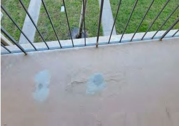
51 Damaged Concrete 2nd Floor Between Units 503 & 504 Overview
