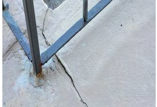
36 Cracked Walkway Near Right Stairwell
