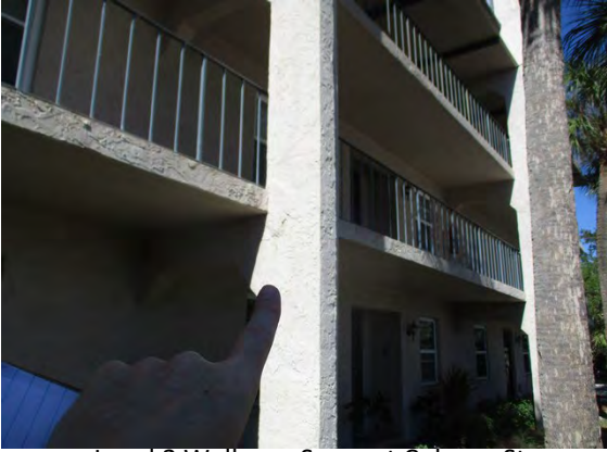
51 Level 2 Walkway Support Column Stucco Cracked/Bulging Between 106 & 107
