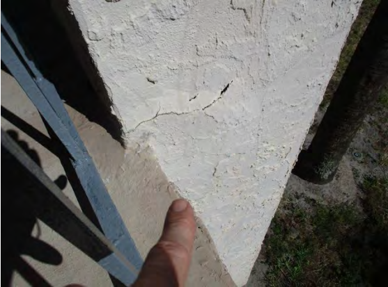
35 Level 2 Walkway Support Column Stucco Cracked/Bulging Right of #206
