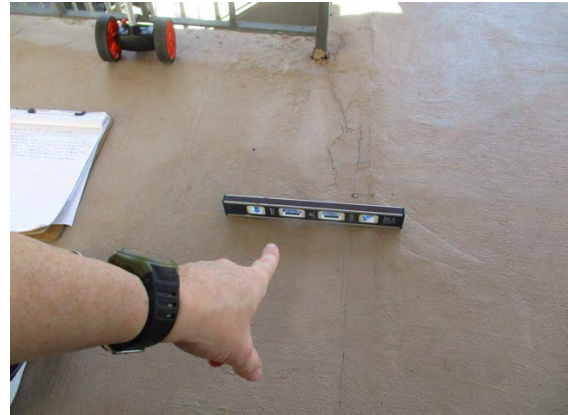
44 Level 2 Walkway Shifted/Displaced/Leaning Left Side of Building
