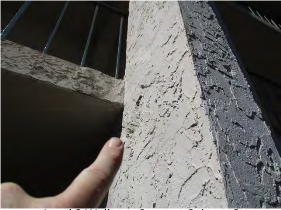
49 Level 2 Walkway Support Column Stucco Cracked/Bulging Between 106 & 107
