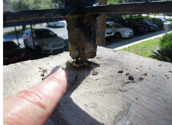
28 Level 2 Walkway Railing Corner Support Post Corroded Through Left Side of Building
