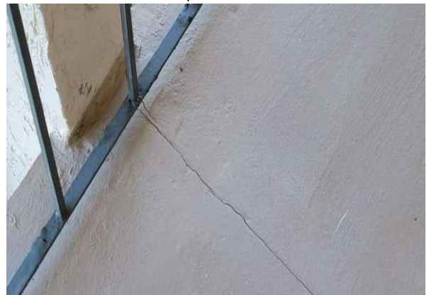
24 Cracked Walkway Near Unit 604
