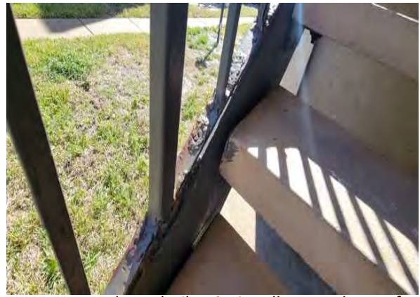
66 Rusted Handrail at Stairwell to 1sr Floor Left Side
