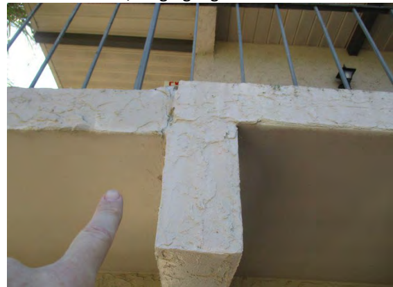
38 Level 2 Walkway shifted/Displaced/Leaning Right Side of Building
