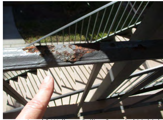
26 Level 2 Walkway Railing Corroded Multiple Areas
