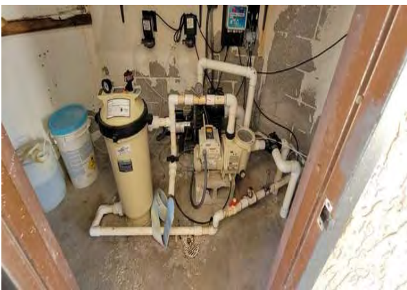
109 Pool and Spa Pumps and Filter
