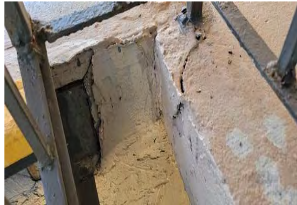
62 Damaged Walkway at Stairwell 2nd Floor Left Side
