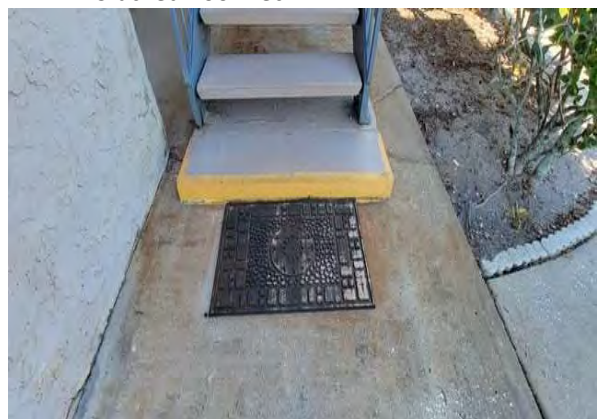
80 Rusted Stair Stringer and Hardware Front Right of Building Overview
