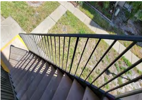
63 Rusted Handrail at Stairwell to 1sr Floor Left Side Overview
