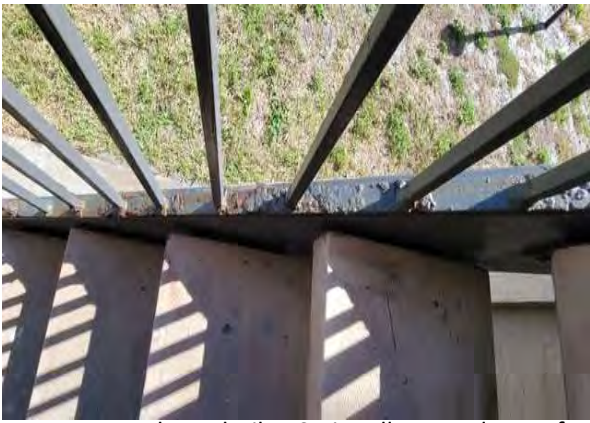
65 Rusted Handrail at Stairwell to 1sr Floor Left Side
