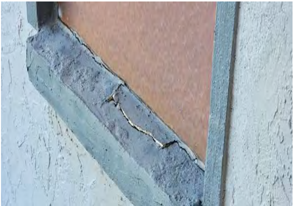
45 Elevator Shaft Decorative Window Sill Damaged
