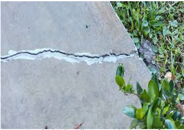
73 Cracked Sidewalk Front Right Corner of Building
