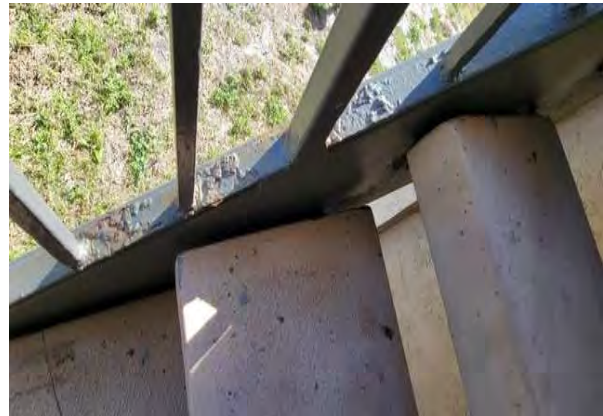
64 Rusted Handrail at Stairwell to 1sr Floor Left Side
