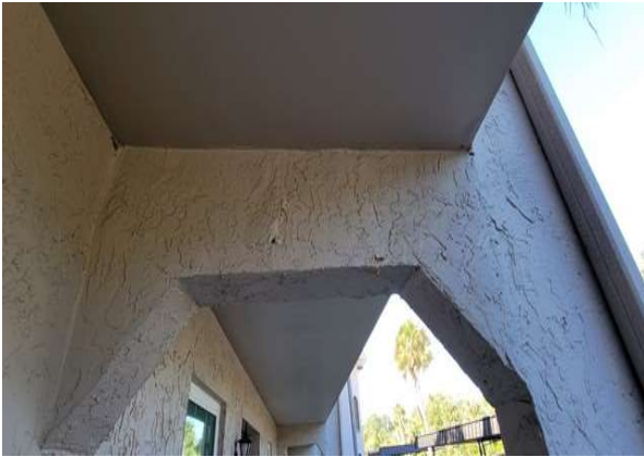
67 Damaged Stucco 1st Floor Near Unit 401 Overview
