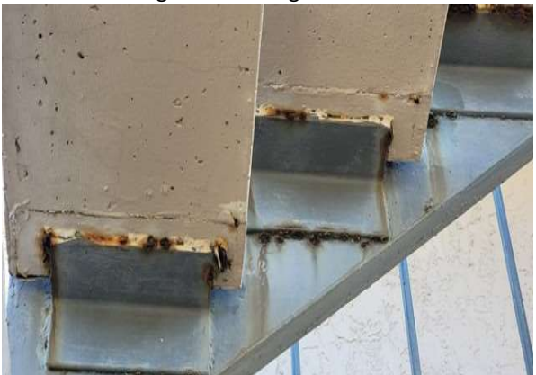
85 Rusted Tread Supports Stairs to 2nd Floor Front Right of Building
