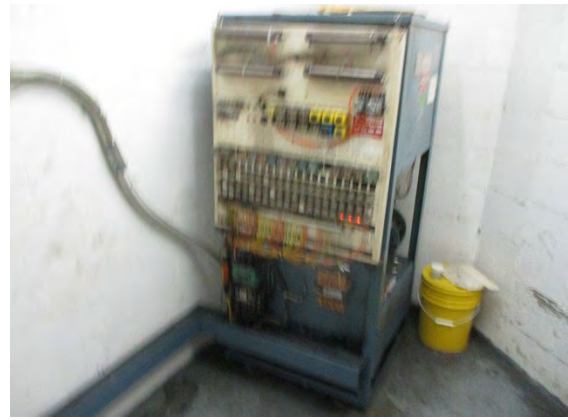
10 Elevator Control Board
