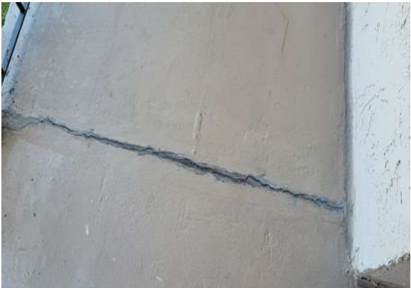
47 Cracked Walkway 2nd Floor Left of Elevator Lobby
