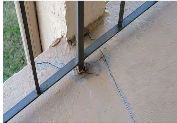
28 Cracked Walkway Near Elevator Lobby 3rd Floor
