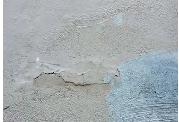
52 Damaged Concrete 2nd Floor Between Units 503 & 504
