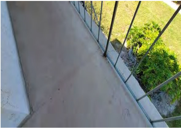
13 Cracked Walkway 3rd Floor Near Unit 608 Overview
