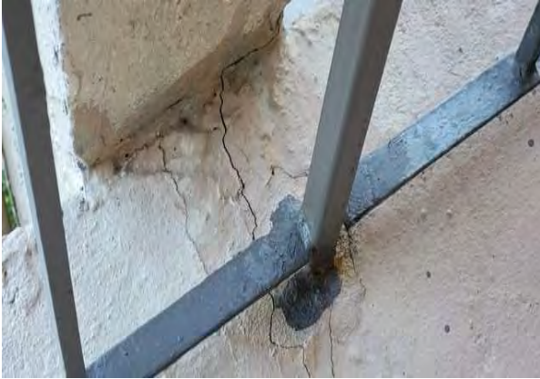
43 Cracked Walkway 2nd Floor Near Unit 504
