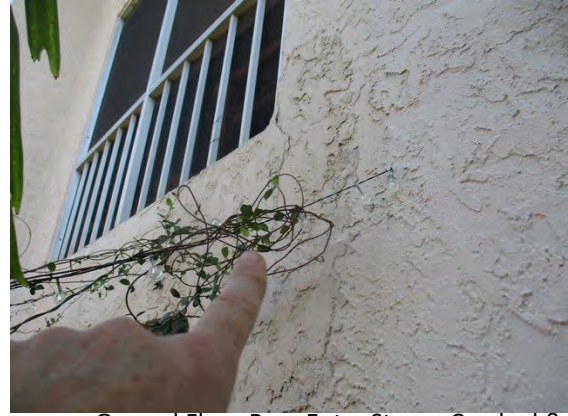
52 Ground Floor Rear Entry Stucco Cracked & Bulging
