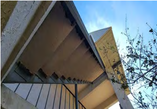
83 Rusted Tread Supports Stairs to 2nd Floor Front Right of Building Overview
