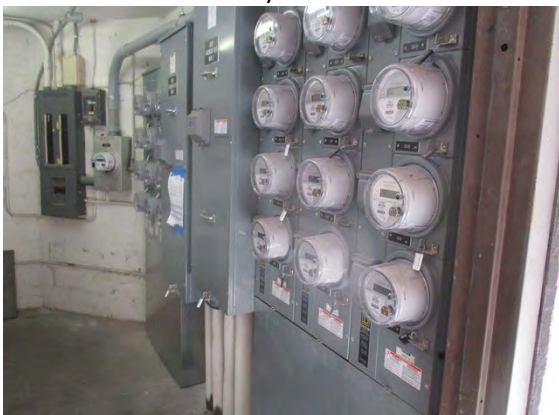
7 Meters & Main Panels
