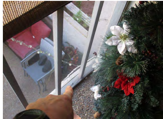
6 Unit 207 Stucco Cracked/Bulging
