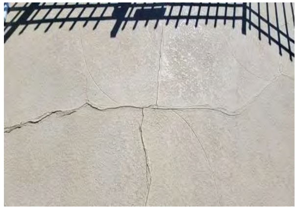
78 Cracked Pool Deck
