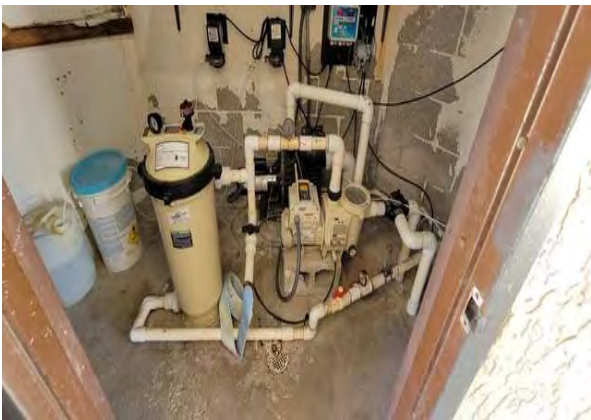
109 Pool and Spa Pumps and Filter
