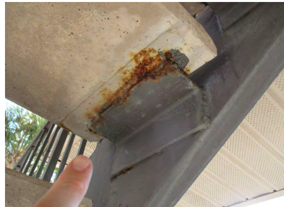
22 Right & Left Stairwell L-brackets For Stair Treads Corroded
