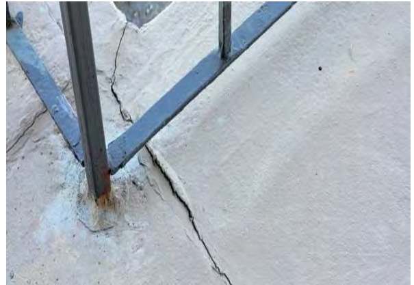
36 Cracked Walkway Near Right Stairwell
