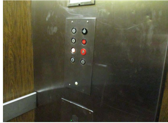
18 Elevator Cab Control Panel
