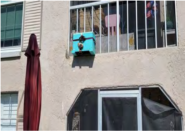
75 Cracked Stucco Rear Wall Between Units 401 & 501 Overview
