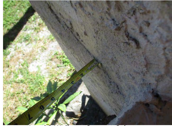
34 Level 2 Walkway Support Column Shifted/Displaced ~1" Left of #202
