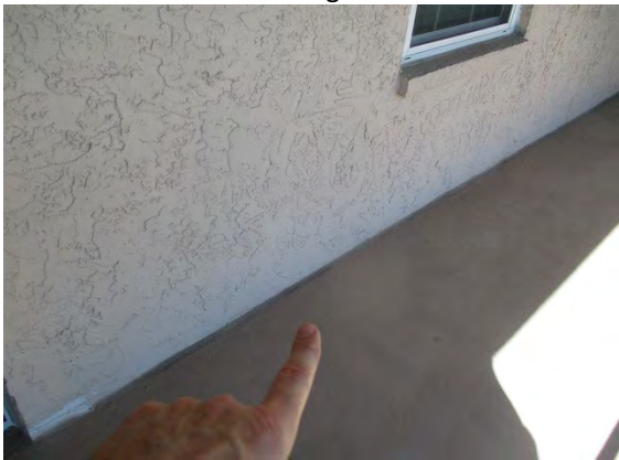
45 Level 2 Prior Repair For Separation at Walkway to Building Connection (Leaning)
