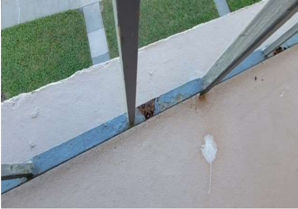
19 3rd Floor Rusted Rail
