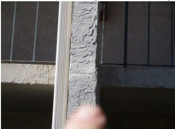
47 Level 2 Walkway Support Column Shifted/Displaced Between 101 & 102
