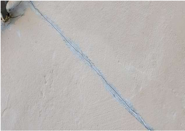
27 Cracked Walkway Near Elevator Lobby 3rd Floor
