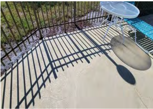
77 Cracked Pool Deck Overview
