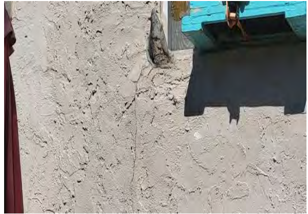
76 Cracked Stucco Rear Wall Between Units 401 & 501
