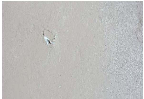
56 Damaged Concrete 2nd Floor Between Units 503 & 504
