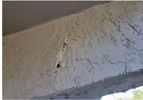
68 Damaged Stucco 1st Floor Near Unit 401
