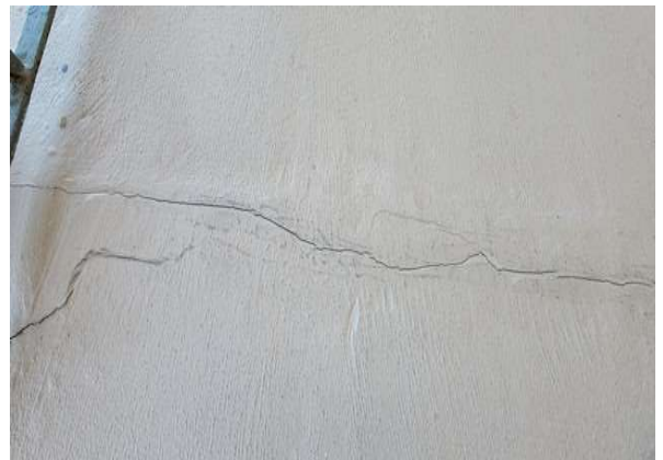
22 Cracked Walkway Near Unit 606
