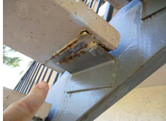
20 Right & Left Stairwell L-brackets For Stair Treads Corroded
