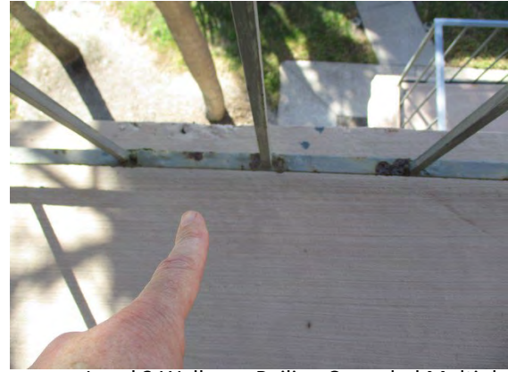
Level 3 Walkway Railing Corroded Multiple Areas
