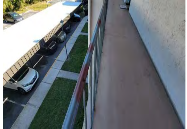
20 3rd Floor Rusted Rail
