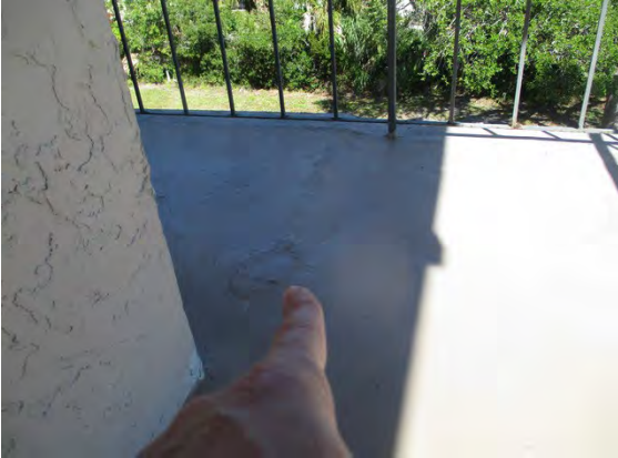
Level 3 Walkway Settled/Leaning At Right Side of Building
