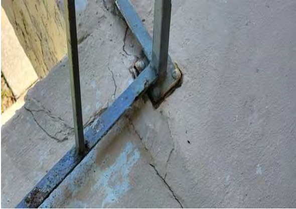
59 Cracked Walkway 2nd Floor Near Left Stairwell
