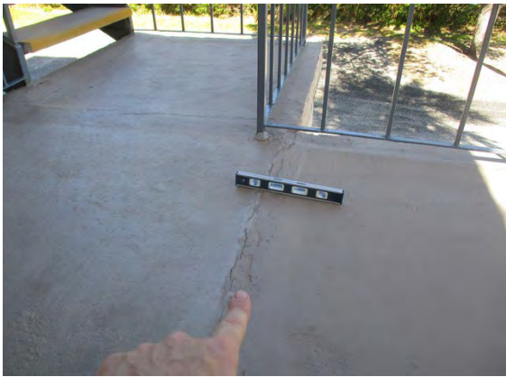
41 Level 2 Walkway Shifted/Displaced/Leaning Right Side of Building
