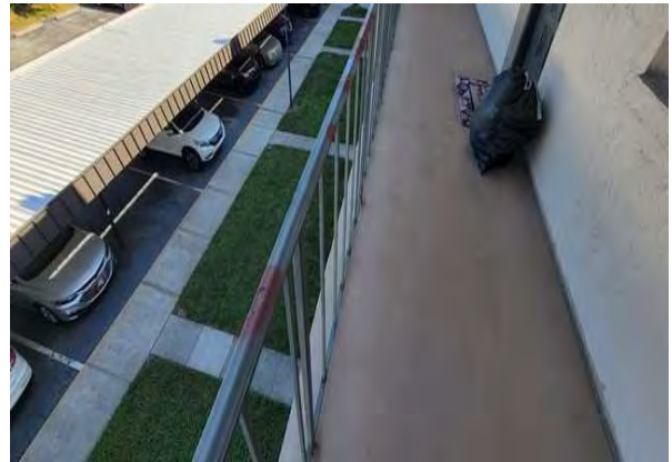
16 3rd Floor Rusted Rail Overview
