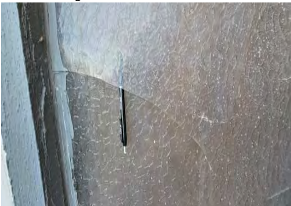
71 Broken Decroitive Window at 1st Floor Lobby Right Side
