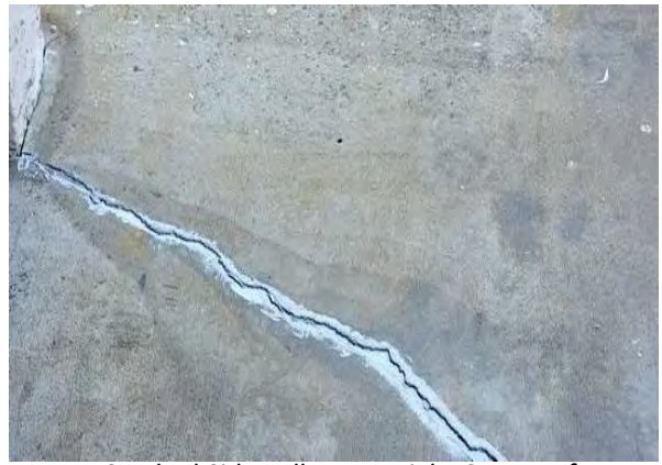
74 Cracked Sidewalk Front Right Corner of Building
