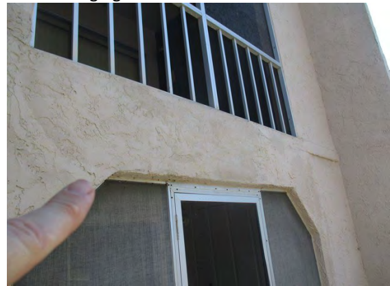
54 Ground Floor Rear Entry Stucco Cracked & Bulging
