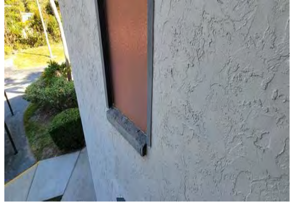
44 Elevator Shaft Decorative Window Sill Damaged Overview
