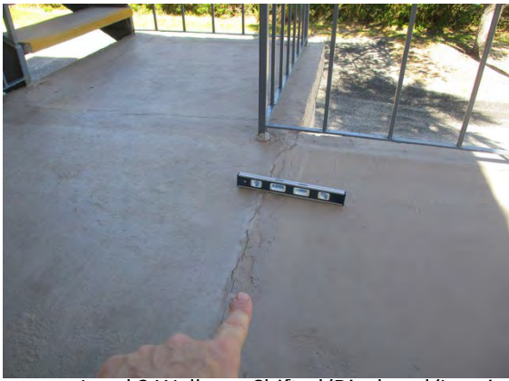
41 Level 2 Walkway Shifted/Displaced/Leaning Right Side of Building
