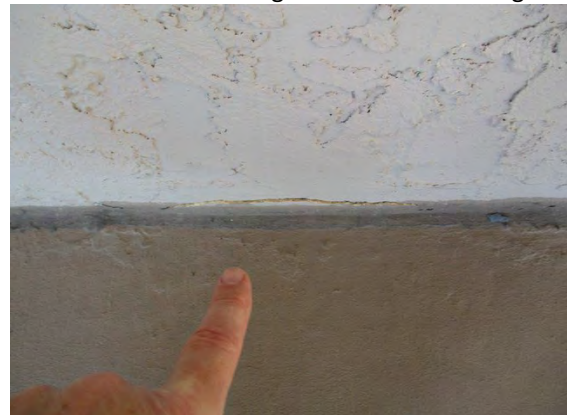
30 Level 2 Prior Repair For Separation at Walkway to Building Connection (Leaning)
