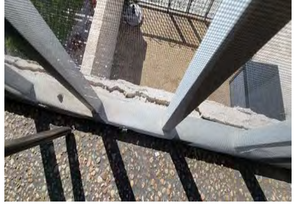
12 Unit 503 Cracked Balcony
