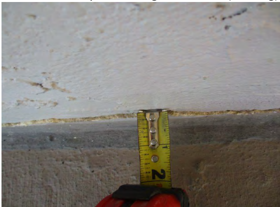
31 Level 2 Prior Repair For Separation at Walkway to Building Connection (Leaning)
