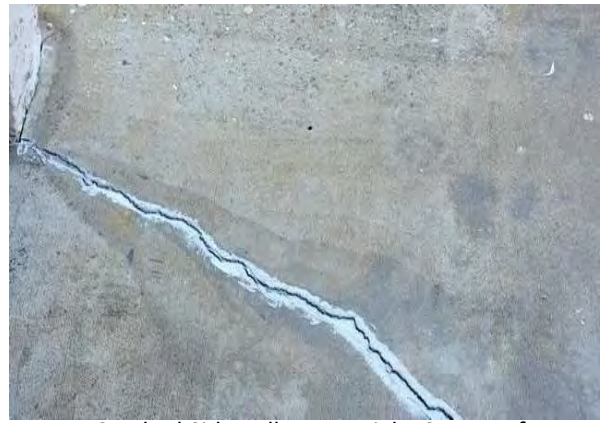
74 Cracked Sidewalk Front Right Corner of Building
