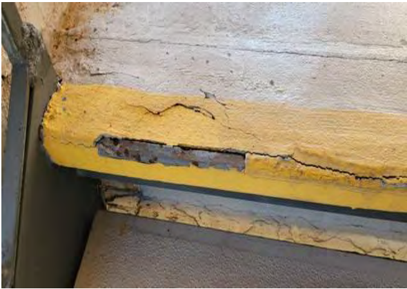
61 Damaged Walkway at Stairwell 2nd Floor Left Side
