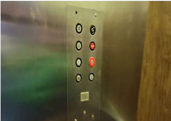
103 Elevator Floor Selection
