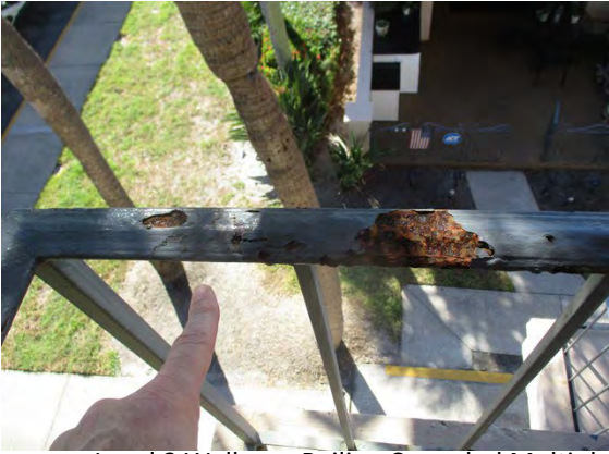
Level 3 Walkway Railing Corroded Multiple Areas
