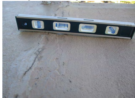
40 Level 2 Walkway Shifted/Displaced/Leaning Right Side of Building
