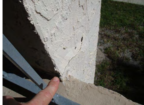
36 Level 2 Walkway Support Column Stucco Cracked/Bulging Right of #206
