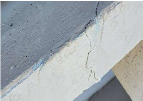
15 Cracked Walkway 3rd Floor Near Unit 608
