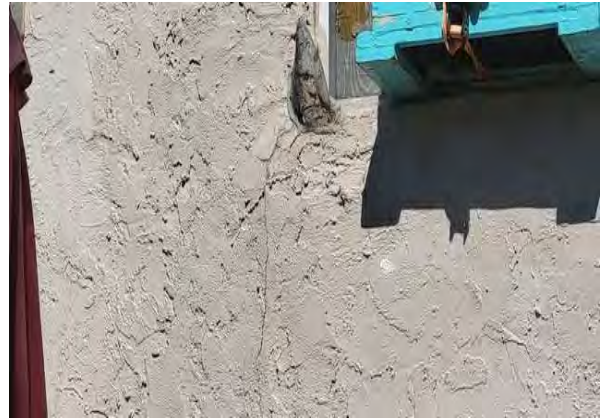
76 Cracked Stucco Rear Wall Between Units 401 & 501
