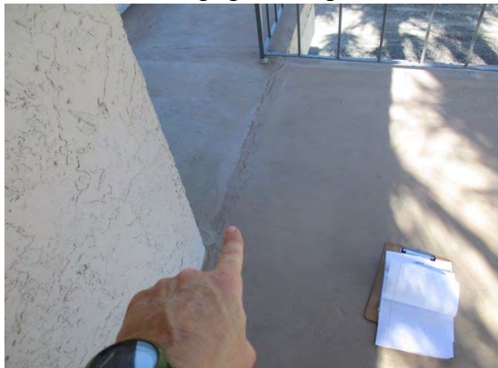
39 Level 2 Walkway Shifted/Displaced/Leaning Right Side of Building
