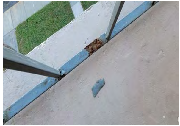
18 3rd Floor Rusted Rail
