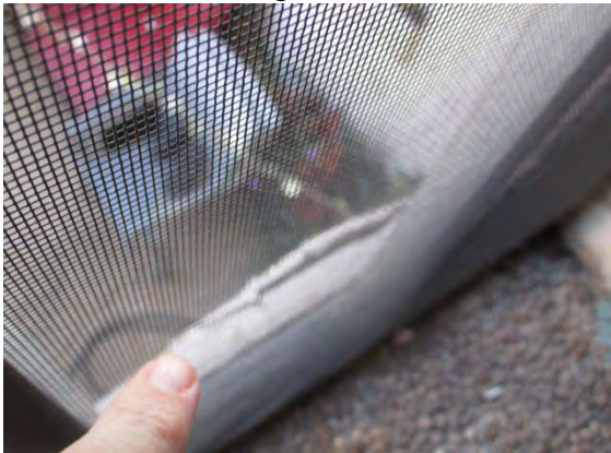
5 Unit 207 Stucco Cracked/Bulging
