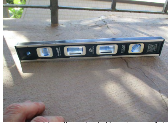
18 Level 3 Walkway Settled/Leaning At Left Side of Building
