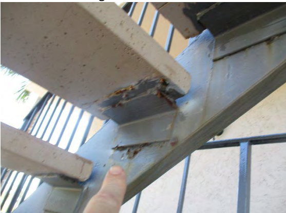
21 Right & Left Stairwell L-brackets For Stair Treads Corroded
