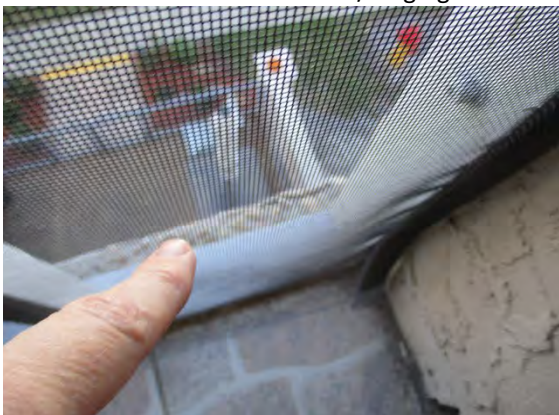
7 Unit 308 Stucco Cracked/Bulging
