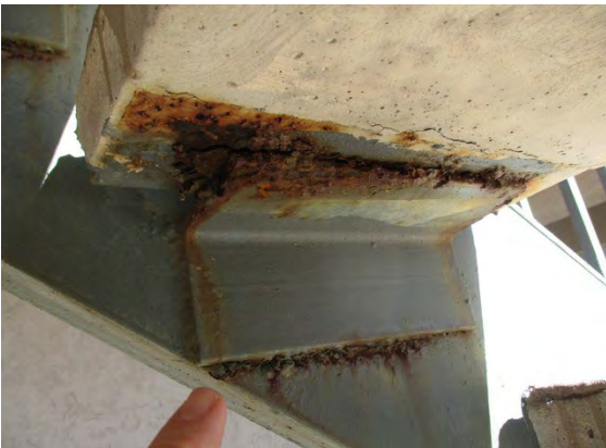
23 Right & Left Stairwell L-brackets For Stair Treads Corroded
