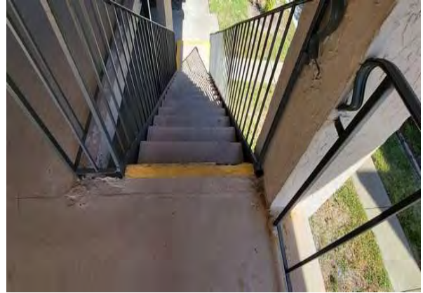
60 Damaged Walkway at Stairwell 2nd Floor Left Side Overview
