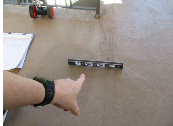
44 Level 2 Walkway Shifted/Displaced/Leaning Left Side of Building
