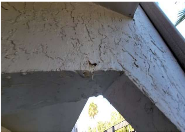
69 Damaged Stucco 1st Floor Near Unit 401
