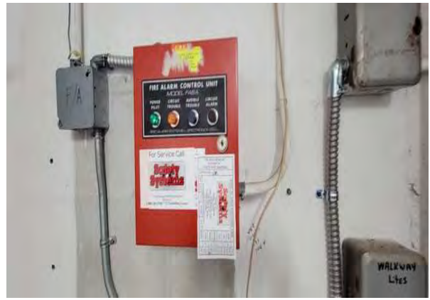
90 Fire Alarm Control Unit
