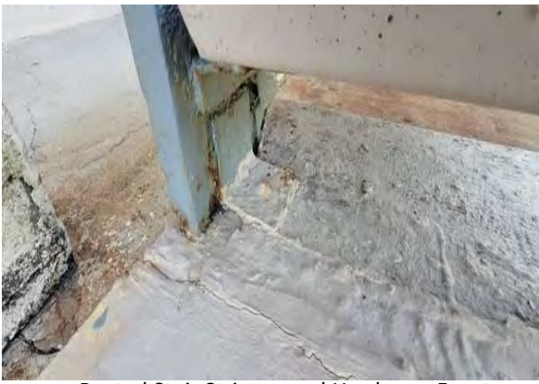
81 Rusted Stair Stringer and Hardware Front Right of Building
