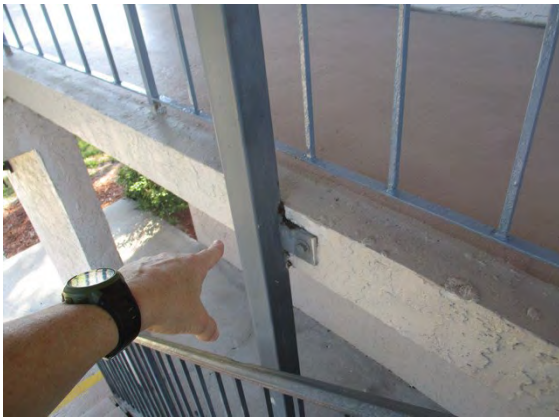
25 Right Stairwell Support Column Corroded
